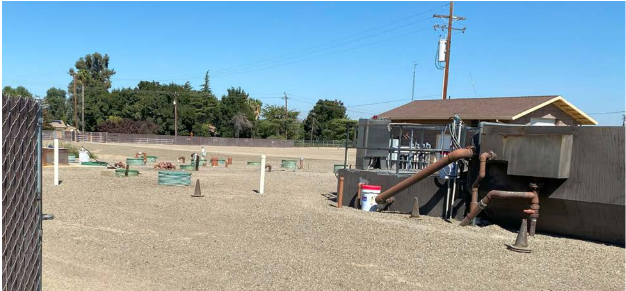
Wastewater treatment plant for CSA 44, Zone G (Linne Estates) Taken Oct 2, 2024
