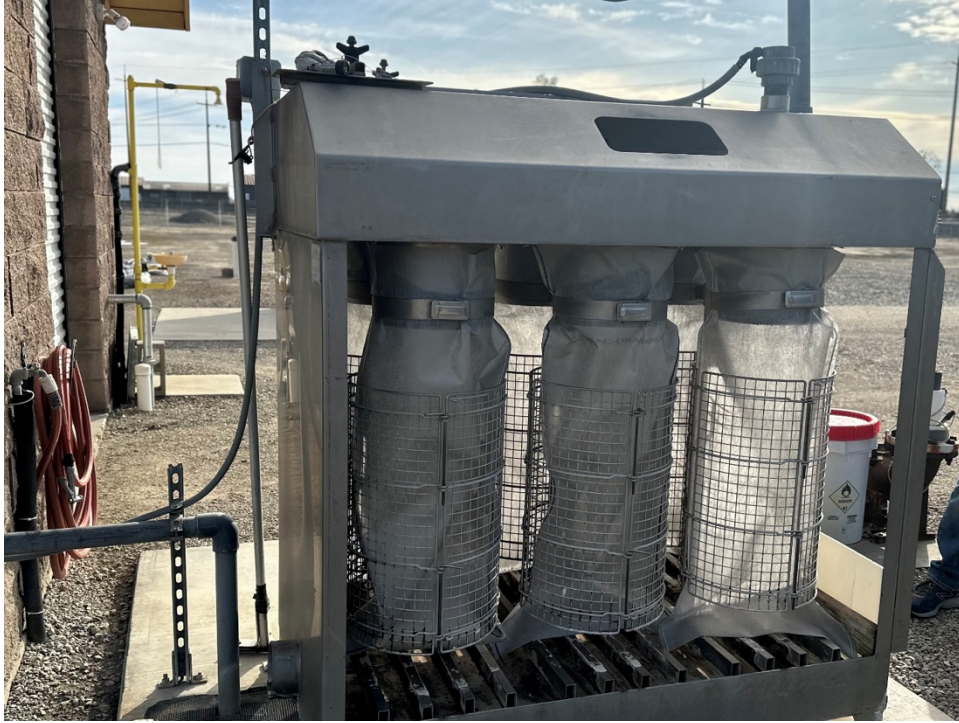
Taken February 21, 2025, bagging stations for bio-solids draining
