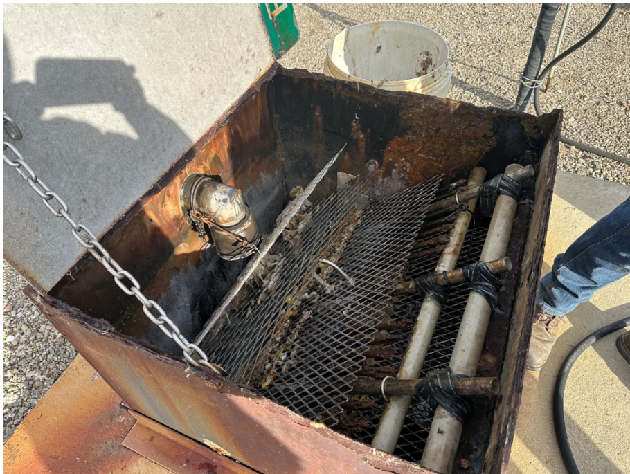
Taken February 21, 2025, bar screen held together with straps and ties
