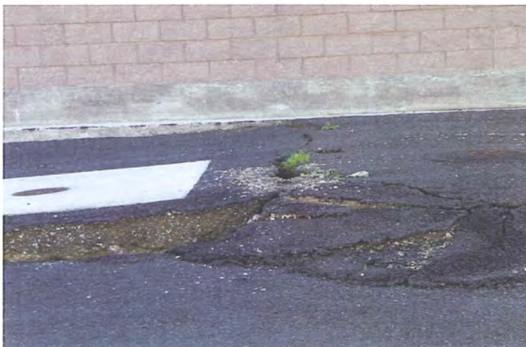
Buckled asphalt at the Intake Pump Station caused by settling ground.Ú
