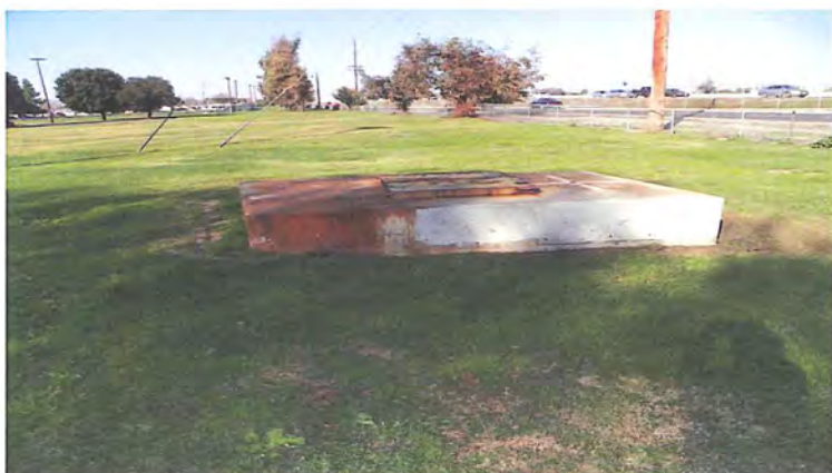
A corroded utility vault in Van Buskirk Park
