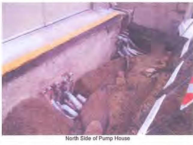
Electrical repairs necessitated by ground settling on the north side of the IPS pump house. Source: Bid Request - Delta Water Supply Project, Intake Pump Station
